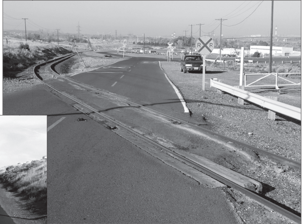
Angled railroad crossing with damaged flangeways on Devore Road at base of hill.
