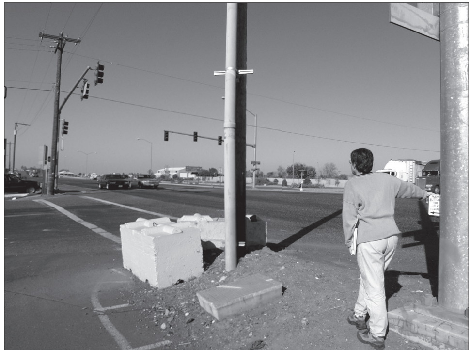
Inaccessible crosswalk on Highway 730 west of I-82.
